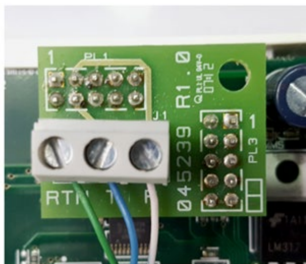
DualCom ION Interface Adaptor situated on the panel
